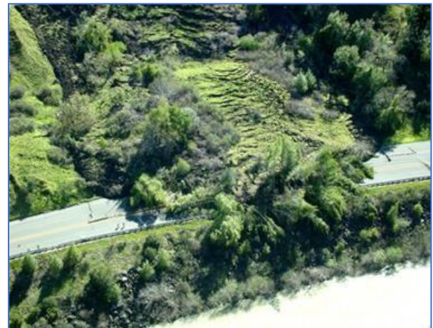
Figure 4.14 Landslide along US 101
