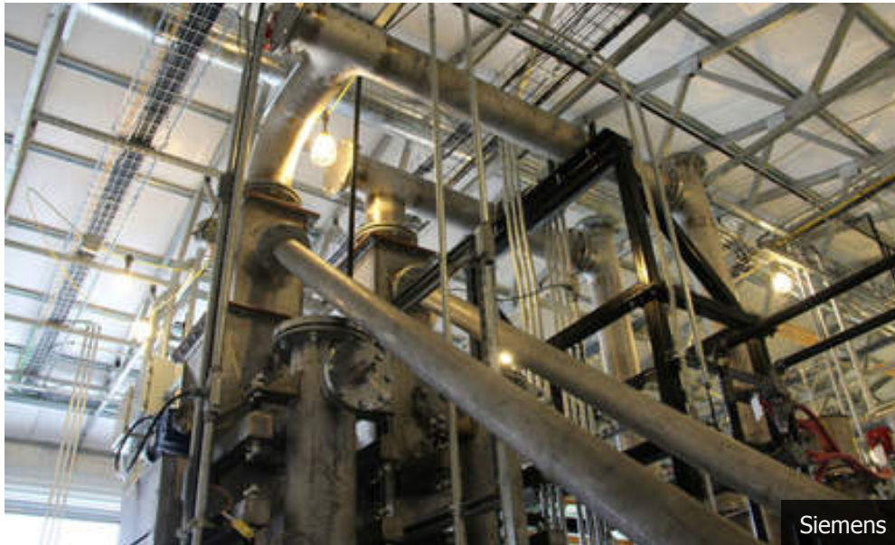
Inside the workings of the Siemens Blue Lake Rancheria microgrid
